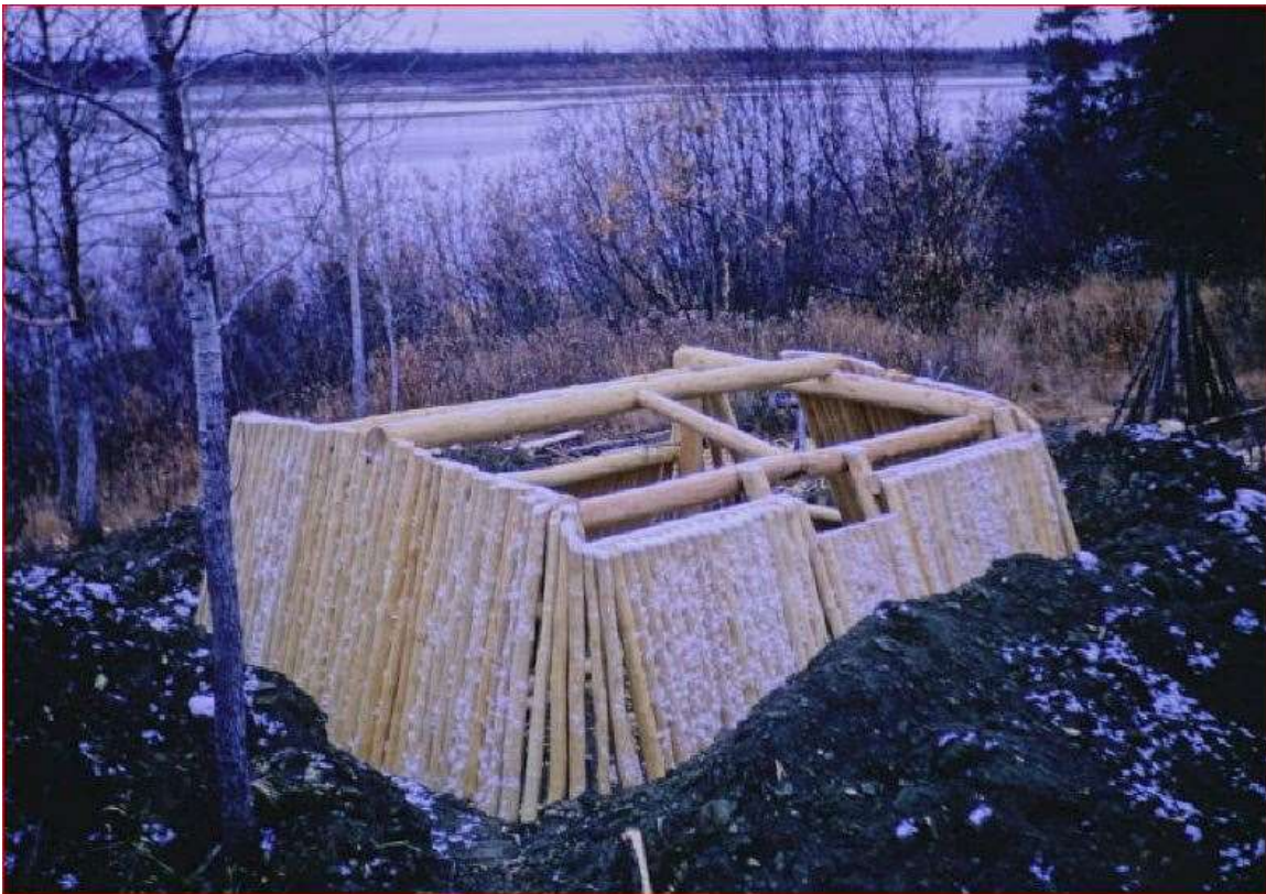
Ole and Sasha made their roof by laying closely spaced poles from the ridge pole to the girts. They left a space in the center of the back wall for the stovepipe safety, and two more spaces for skylights. Image: Sasha Wik
