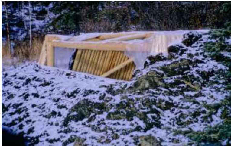
Ole and Sasha backfilled the walls before building the roof in order to prevent the piles of dirt from being covered by snow. Image: Sasha Wik
