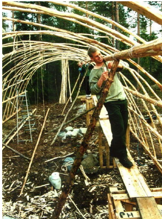
Trond Pedersen helps attach a horizontal member to the half-circle frames. Image: Rein Dammann
